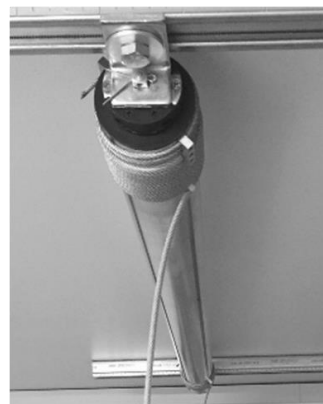
Even without tension the cable wraps are neatly side by side and no overlapping.
