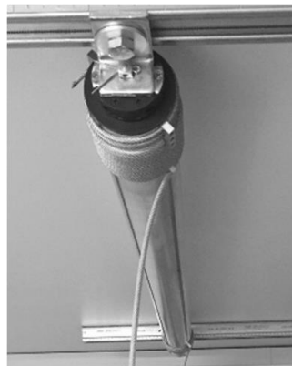
Even without tension the cable wraps are neatly side by side and no overlapping.
