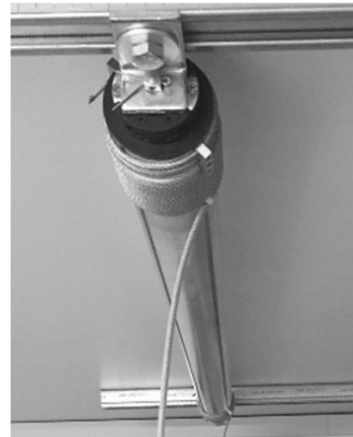
Even without tension the cable wraps should be side by side and there is no overlapping.
